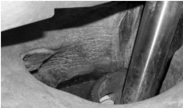
Slika 2: Poškodba reaktorske glave v elektrarni Davis Besse Figure 2: Damage on Davis Besse reactor vessel head
