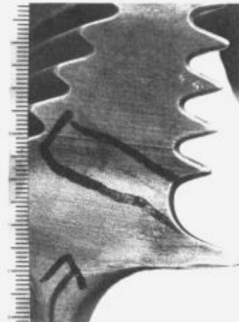
Figure 1: Crack on the trailing edge in the first root groove of blade 436.
